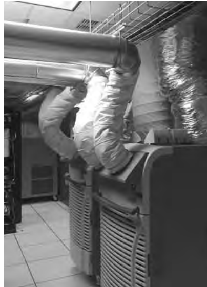
The use of 5-ton MovinCools with flex/overhead ducting provides emergency cooling in any area where it's needed.
