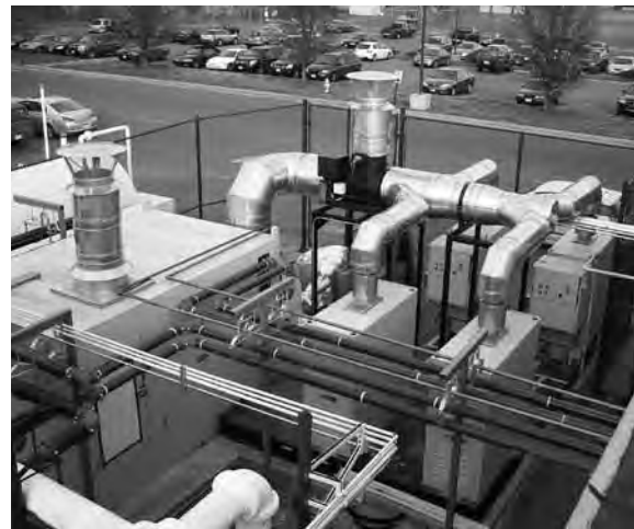
A view of the new CCHP system workings at Branford High School.
