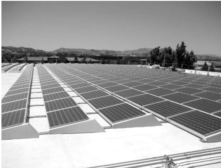
A view of the PV panels installed at the Pleasanton, CA facility.
