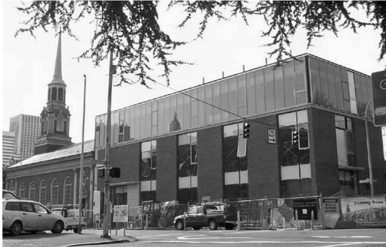
Construction in progress on the First Unitarian Church of Portland's LEED-certified building.
