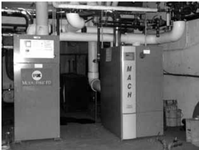
Modulating boilers replaced a broken system, saving an estimated $7,200/year in heating costs.
