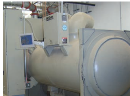
Fully EMS-compatible chillers at Frontier High School.
